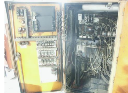
A control panel door left open to prevent over-heating
