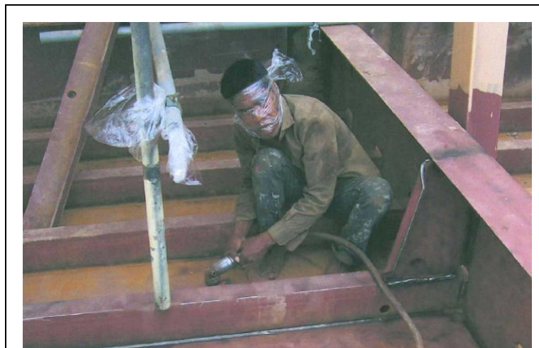
External engineer using dangerously inappropriate protection equipment
