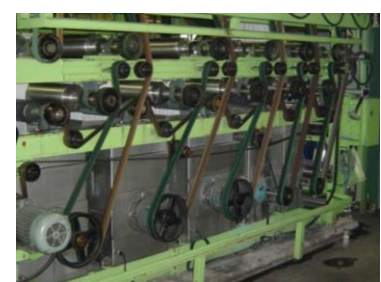
Unguarded cogs on a continuous wash range: Pose an unacceptable risk
