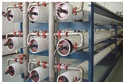
Reverse Osmosis System
