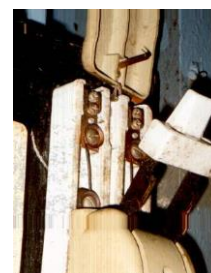
Old fashioned, exposed electrical circuitry are a serious risk
